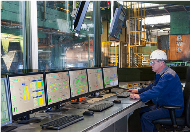
Reference: V7 Control room
